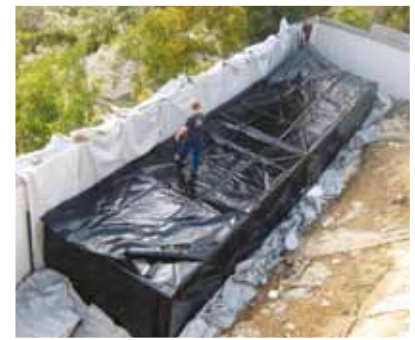
CelluTank® Re-use System Eaglemont Victoria.
